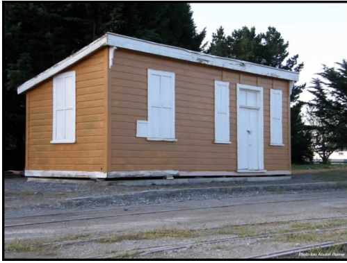
Waingawa Station seen after first coat of new paint Photo Iain Alisdair Palmer
